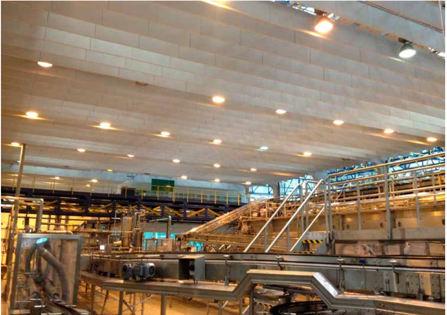
Almost 2,000 sound absorbing baffles provide an acoustic environment that is acceptable for the employees and that meets the legal requirements at the Danang brewery.
