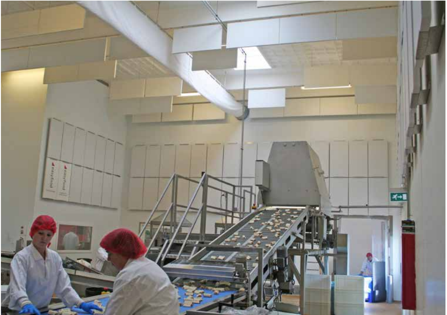
In the ceiling, sound-absorbing baffles in combination with an anti-corrosion system of wall absorbers. The total area of sound absorbers is almost twice what it was before. It is now easier for the staff to communicate with each other in a normal tone.
