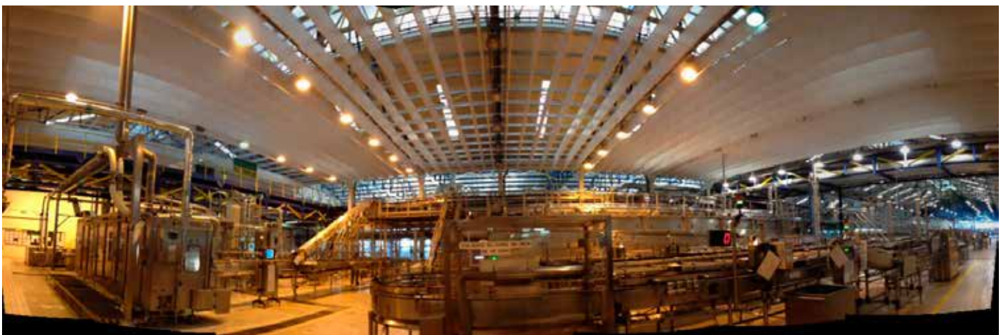
Two lines at APB's brewery in Ho Chi Minh City, one opened in 2009 and the other in 2011. The brewery is the fastest and most advanced canning lines in Vietnam. Tiger and Heineken, beer are produced here.
