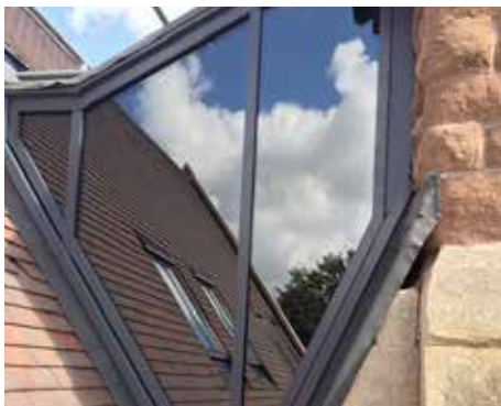
Bespoke vertical glazing, St. Stephens Church, Birmingham
