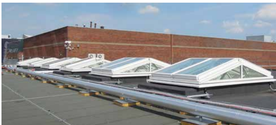
Glazed smoke ventilators installed at the Queens Square Shopping centre, West Bromwich
