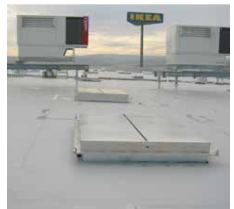
Smoke flap ventilators, IKEA superstore
