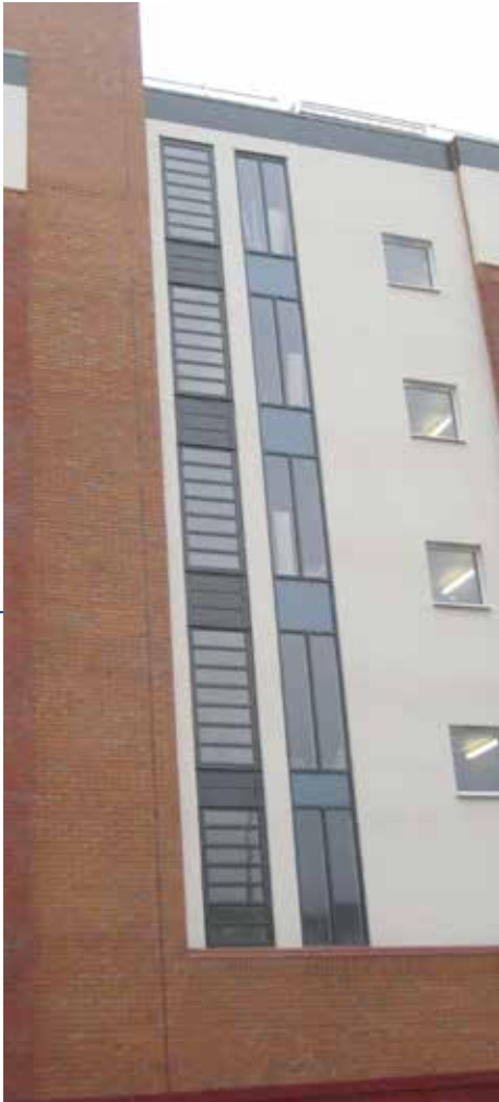
Architectural louvred smoke ventilators combine functionality with integrated aesthetics at this city centre hotel
