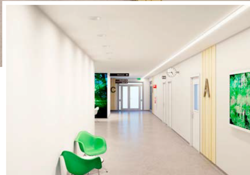
Notor recessed LED offers an unbroken line of general light, with Pleiad G3 Wallwashers providing a higher proportion of vertical light on the adjacent wall.
